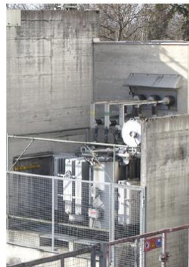
Station service transformer
