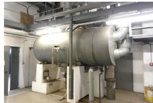
Heat exchanger for district heating
